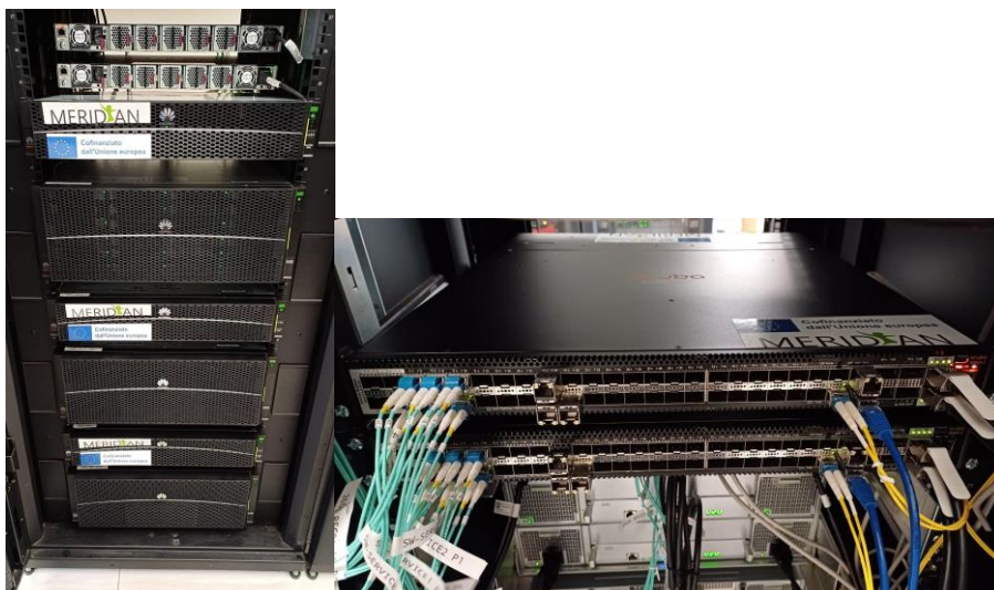
The new storage system
