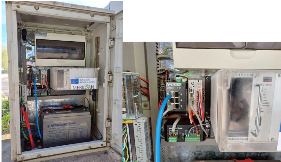
Interior of a legacy traffic data collection station cabinet
