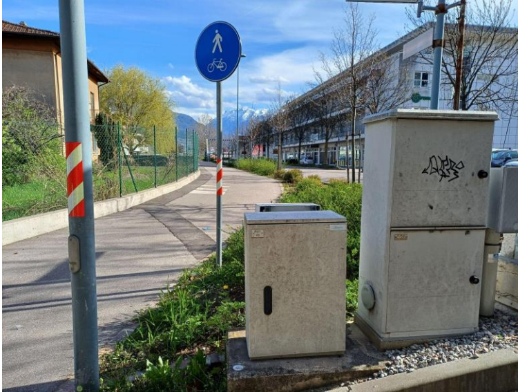
A legacy traffic data collection station cabinet
