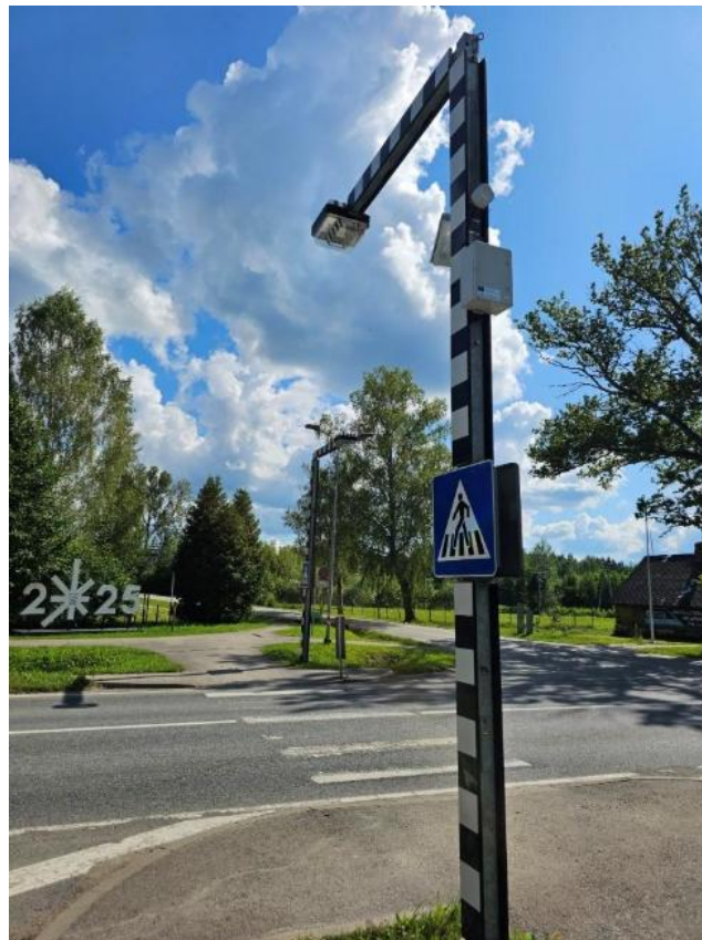
Equipment mounted on pedestrian crosswalk light pole
