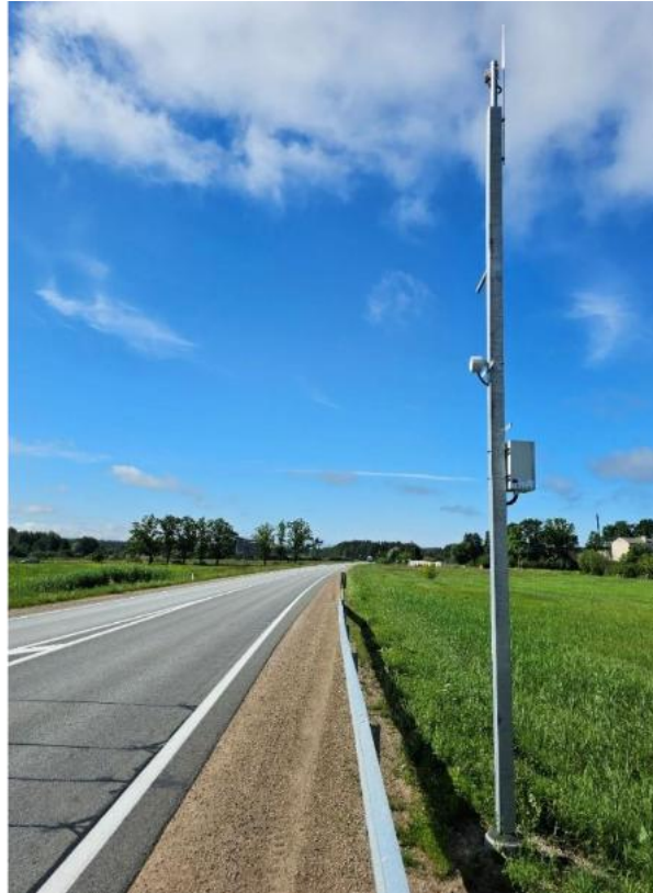
Roadside pole with equipment and road safety barrier
