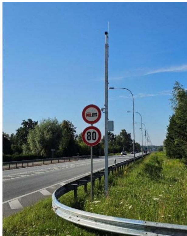
Traffic counting point installation with equipment cabinet, external antenna and traffic counting sensor at the very top of the pole
