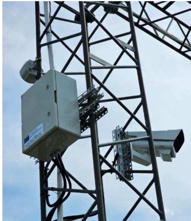
Pedestrian and cyclist counting equipment mounted on traffic light base
