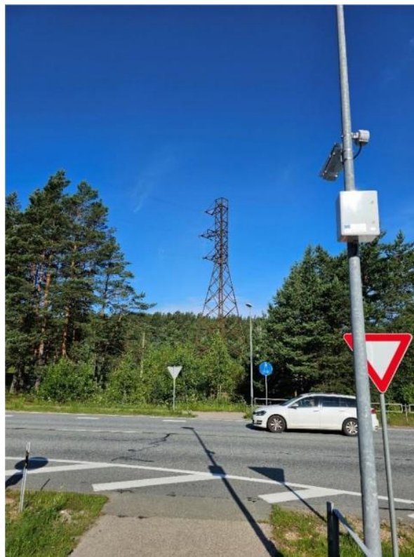
One of the 10 installation locations, with camera, external antenna and cabinet mounted on pedestrian path light pole
