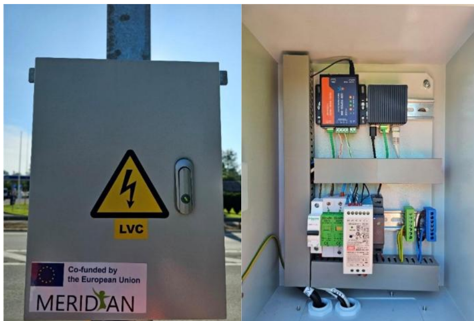
External and internal view of the main traffic counting point cabinet which is mounted on roadside pole
